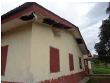
Ronietta CHP before rehabilitation
