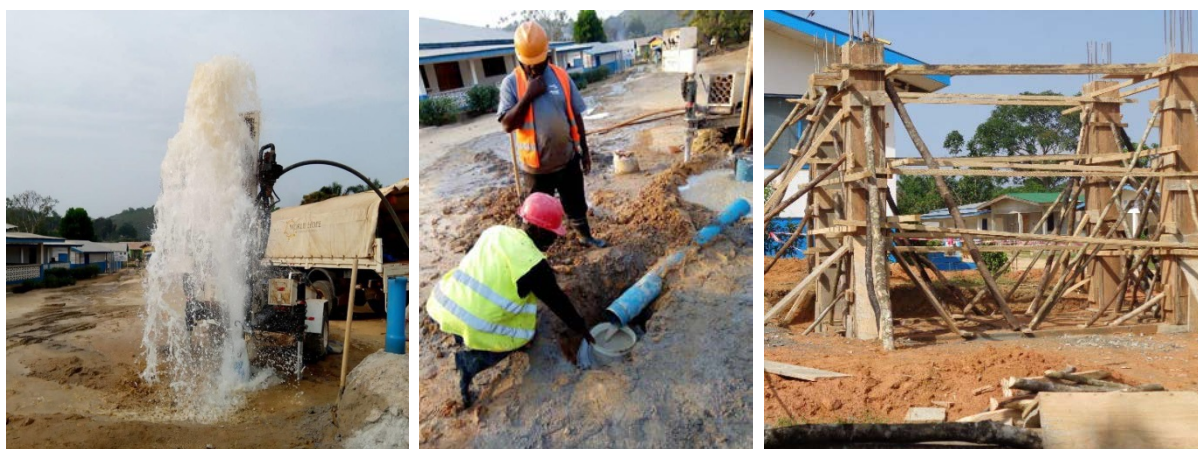
From left to right: Kolahun well development; measuring blow yield during drilling; and cast columns and ground beams for the water tower. Photos: APC
