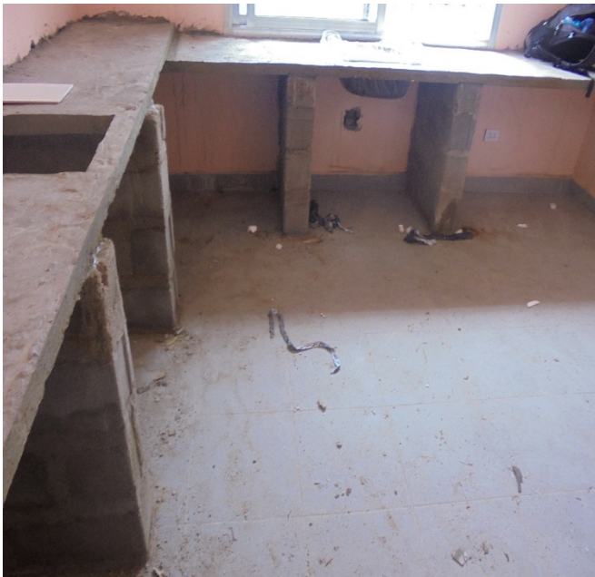
The laboratory at JFK Medical Center Outpatient Infectious Disease Clinic before renovation. Photo: APC.
